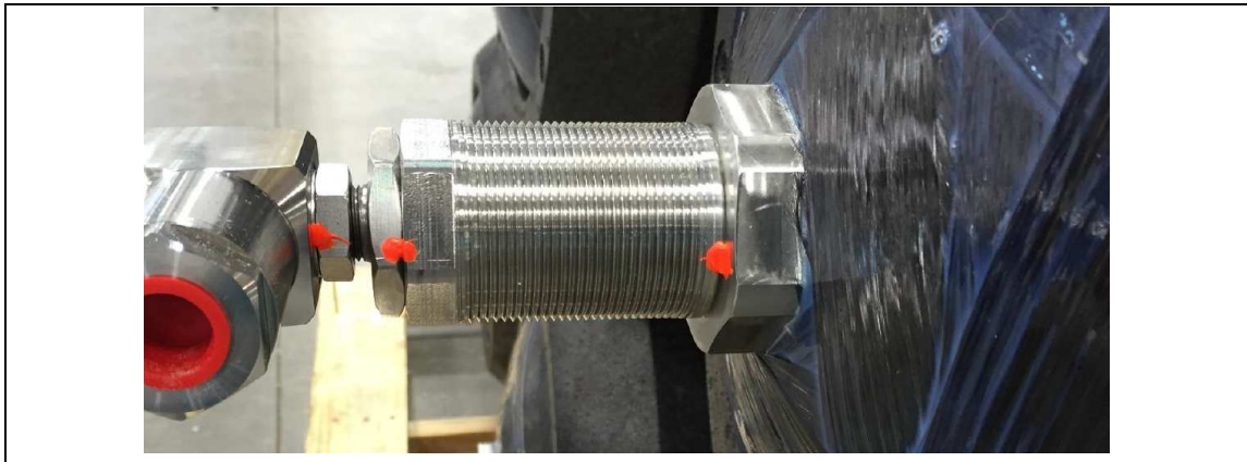
Threaded end of the extender installed on a cylinder. Also visible, red torque markings. .
